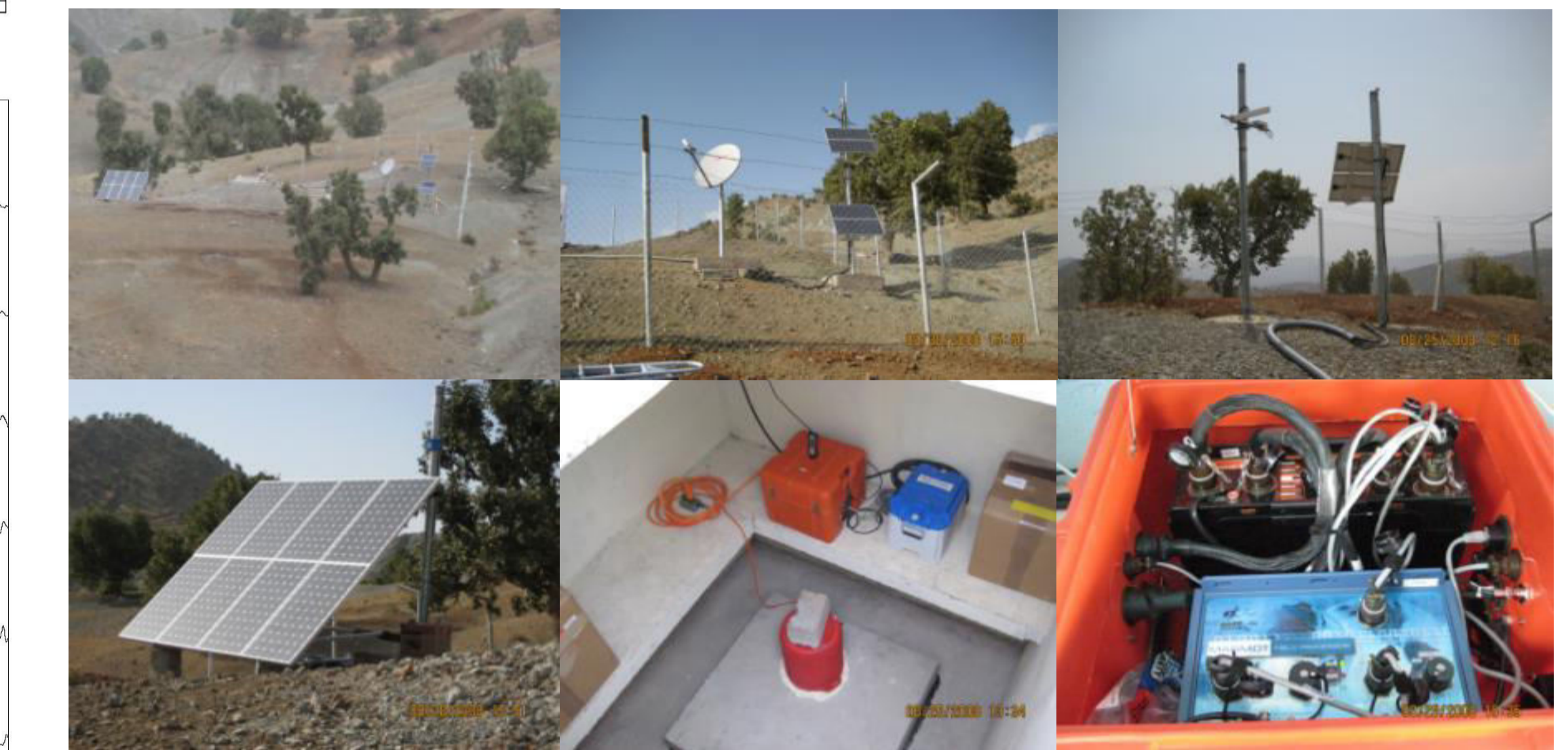
Figure 4. Pictures showing the seismoacoustic array KSIRS station's vaults, instrumentation, radio and satellite communication, and solar power.
