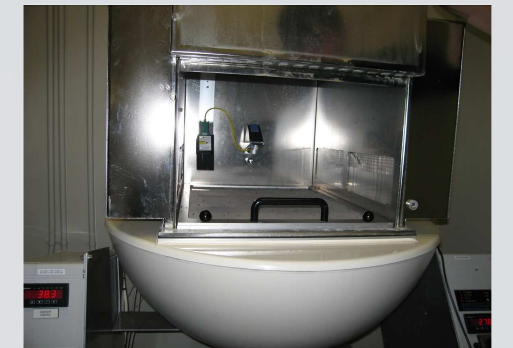
Filter heaters inside the filter chamber St. John's CAP17
