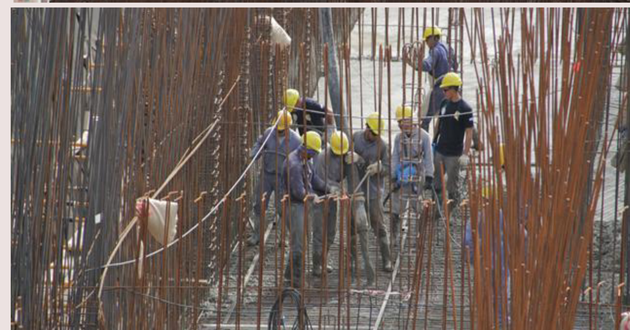
Fig. 1a and 1b: Base of the reactor: 180 trucks poured 1500 m 3 of concrete over 225 ton of iron to complete the concrete slab, the similar amount to raise a building of 10 floor.
