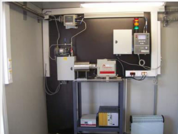
Stack Monitor at IRE
