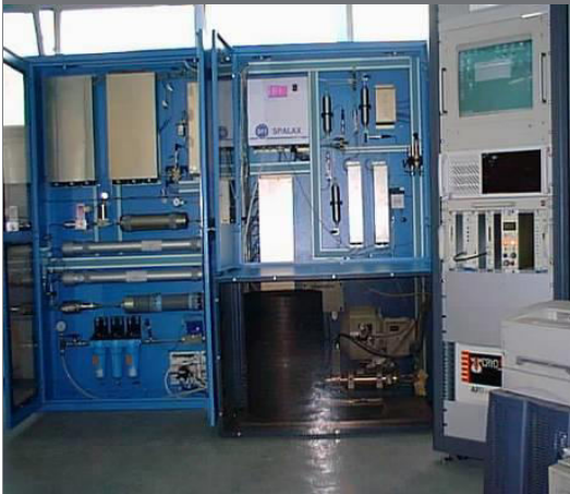
The SPALAX xenon monitoring system uses membrane separation along with germanium gamma spectroscopy
