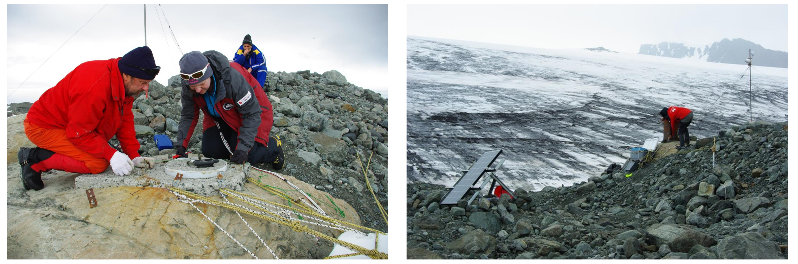
Fig. 1 (left) Installation of seismic station LIVV; (right) Seismic station LIVV and glacier Perunika
