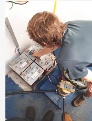
Site-survey and trouble shooting
