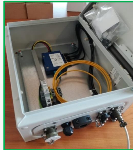
Ethernet cabinet FO Patch cabinet
